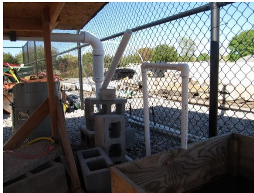
Figure 6. OSU-OKC AS downspout configuration.
