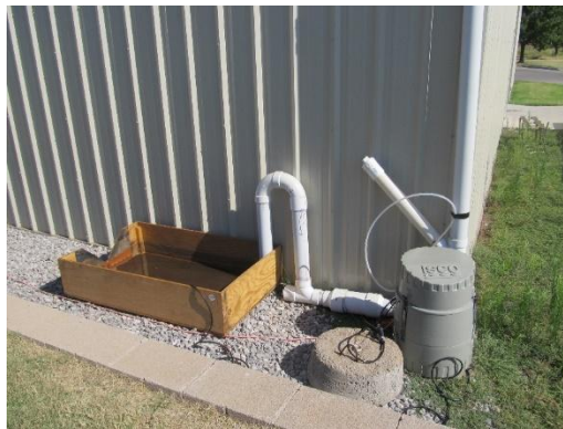
Figure 8. HP downspout setup, including weir box and portable sampler.
