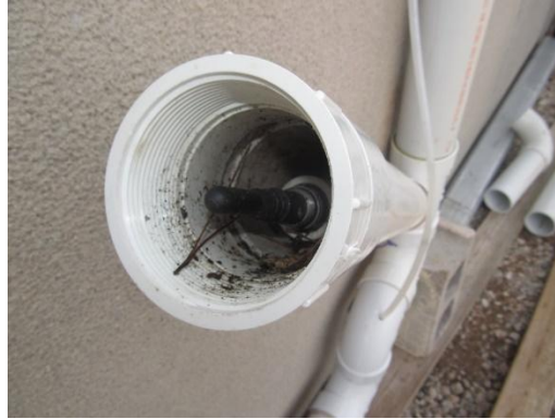
Figure 7. Sonde inside the HP downspout configuration.
