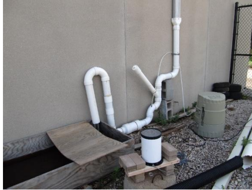
Figure 5. OSU-OKC MS downspout configuration.
